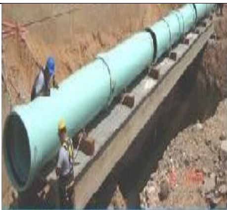
Prog Mgr: 36-inch Sewer Line Construction Over Sinkhole on major Street in Waco, with in-house crews at 50% low bid cost
