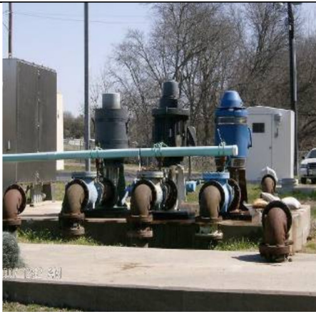
Design Report Mgr: for WWTP Pump Station Upgrade at the City of Azle
