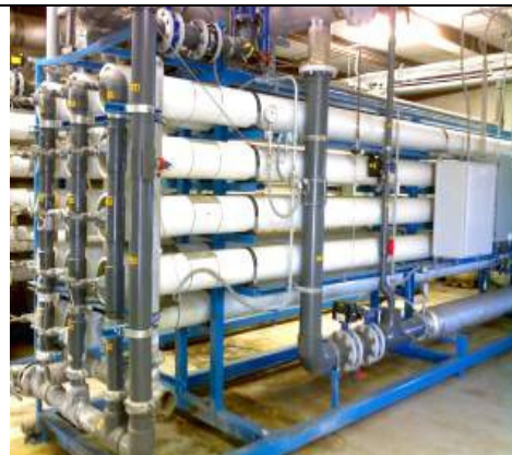
Asset Mgr: Reverse Osmosis Plant
