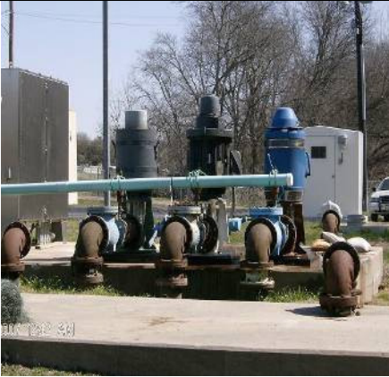
Design Report Mgr: for WWTP Pump Station Upgrade at the City of Azle
