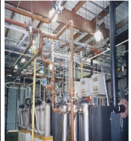
Proj Engr: Kelly AFB Groundwater Chlorinated Solvent UV/H2O2 Reactors Capacity Upgrade
